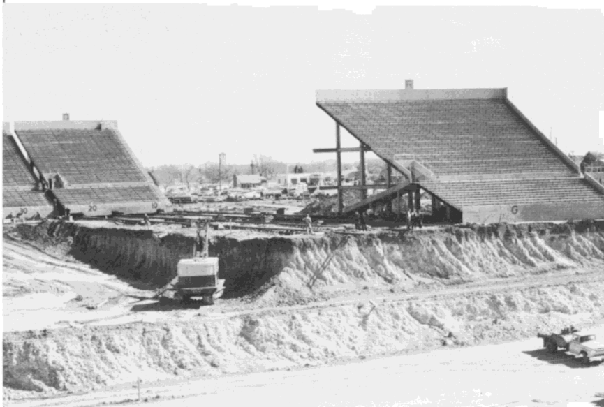
As the east stands were being moved, workmen continued to excavate the playing field during the 1959-60 expansion of Jones Stadium.
