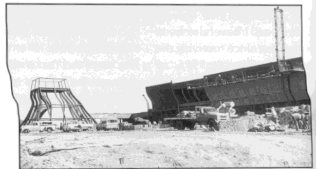
Construction of the new building began in September 1968. At left is the steel skeleton of the Moody Planetarium. (Heritage Club #C198, Southwest Collection)
